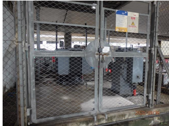
Photo 10. Tsuen Wan Regional Lab Substation
