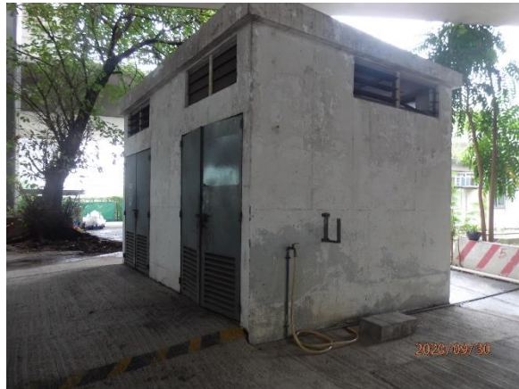
Photo 6. Abandoned Store for Dichloromethane
