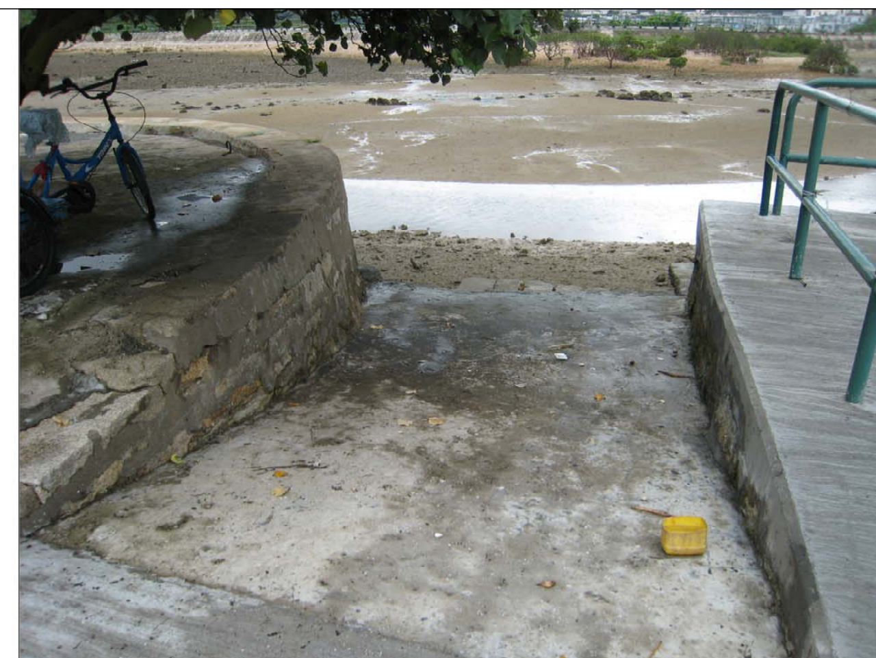
③ EXISTING RAMP TO BE REMOVED AND REINSTATED AFTER CONSTRUCTION 現有斜路會臨時清除並於竣工後恢復原狀
