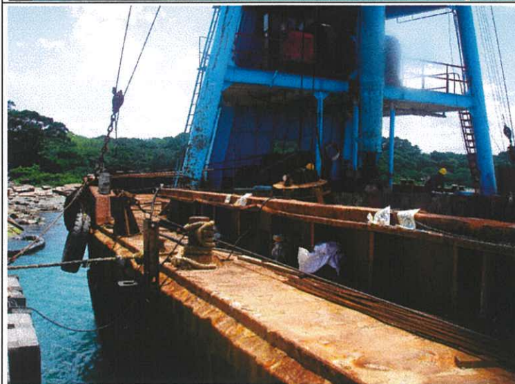
Plate 15. The Work Barge for this project. All material had to be kept in the hold to ensure that nothing could fall onto the corals below.
