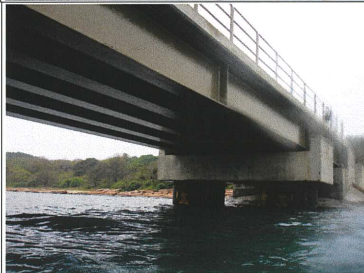
Plate 27. Underneath view of the new pier. The two caissons are shown in this photograph. (April 2007)
