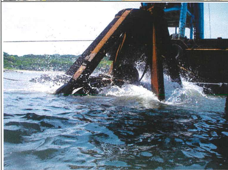
Plate 17. The rock grab in action. Only one day was required for this work.
