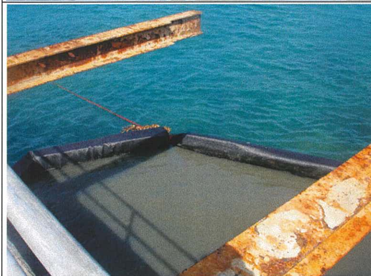
Plate 18. The caisson guides were used to align the grab. Note the effectiveness of the sediment curtain.
