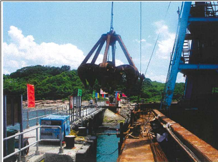
Plate 16. The deeper foundation for the caisson piles was dug using a rock grab. Both surface and in water guiding of this work phase was carried out.
