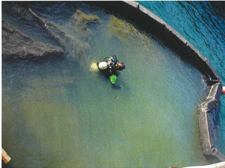
Plate 9. A diver working inside the sediment curtain removing rocks so that the caisson piles could be installed under the pier.
