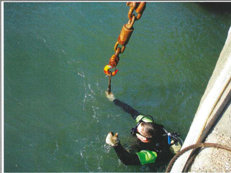
Plate 11. A diver working with the crane operator to remove the rocks around the old pier structure. Some of these rocks weighted nearly one tonne.
