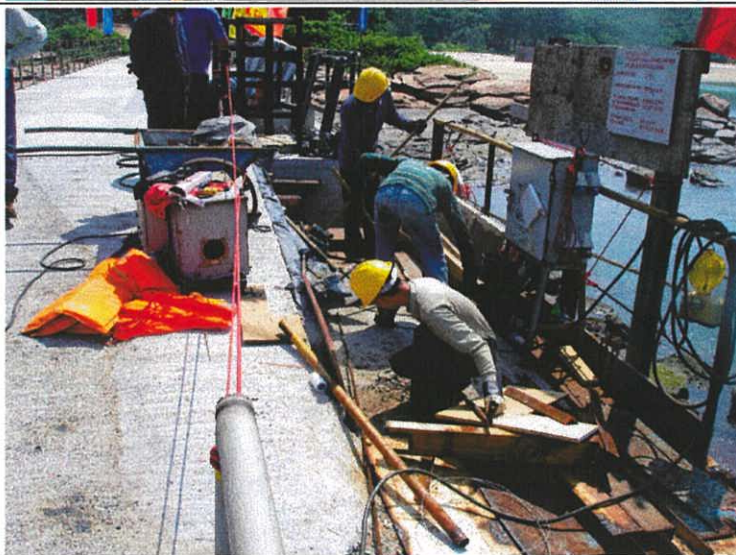
Plate 21. The pier was not closed to the public during this renovation so there were limited areas on the pier for the construction crew to work. This is one such area.
