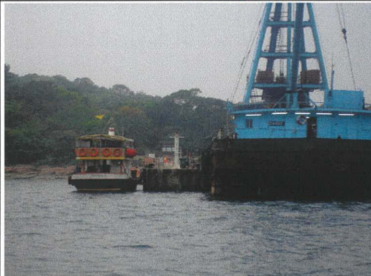
Plate 6. The location of the Works Barge. The addition of this vessel allowed the pier to be kept clear of construction equipment and debris.
