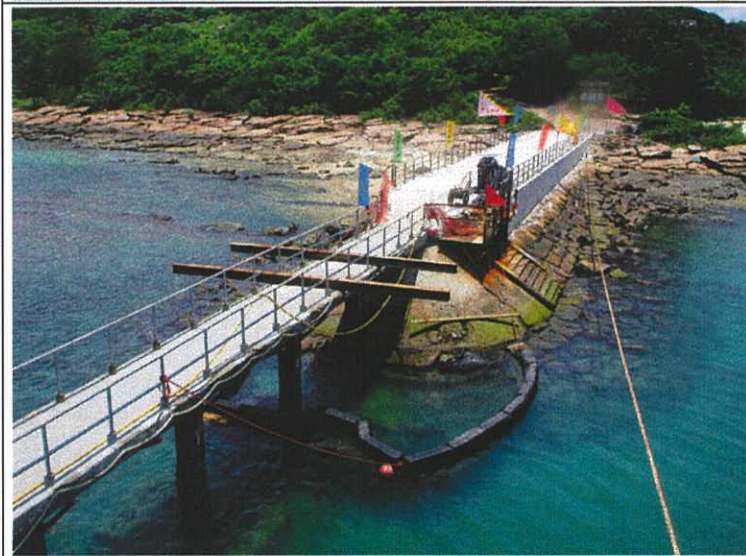
Plate 14. A view of the worksite showing the installation of the guides for the caisson piles.
