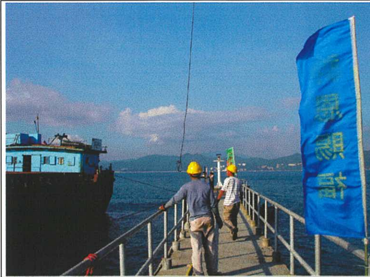
Plate 10. Coordination of the temporary removal of the burnishing stones from the foot of the old pier. These rocks were lifted out one by one.
