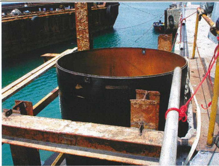
Plate 20. Finally the first caisson goes in. It was gently vibrated through the sand until it reached firm bed-rock.
