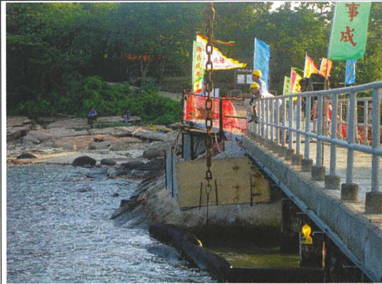
Plate 13. Reinforcing the pier footing to allow it to take the weight of the new pier section.
