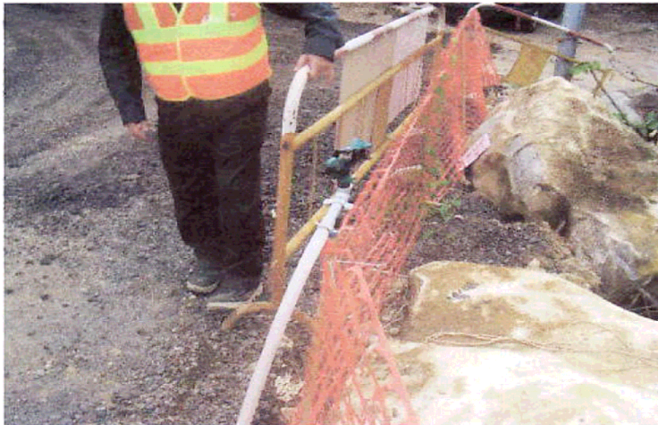
(Fig 3) Water sprinklers were installed for dust suppression, photo taken on 3 rd December 2008
