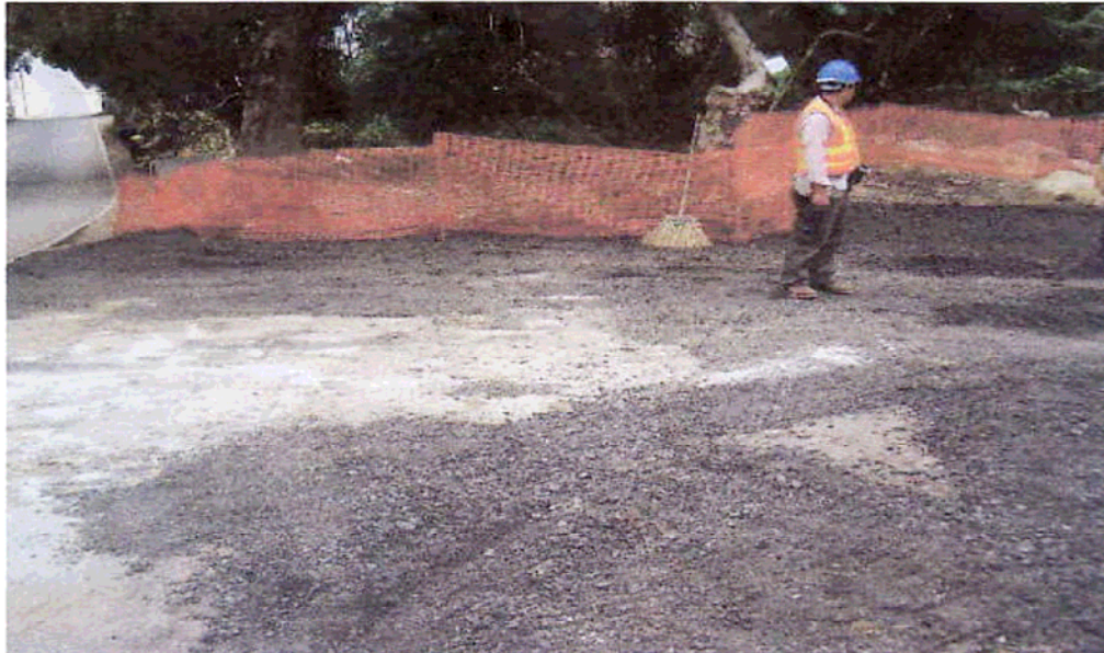
(Fig 1) Site entrance was paved with bituminous materials, photo taken on 3 rd December 2008
