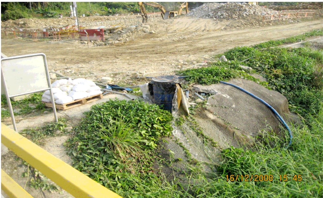
Fig.4 Defective desilting facilities found at LTR road B ch.950~1000
