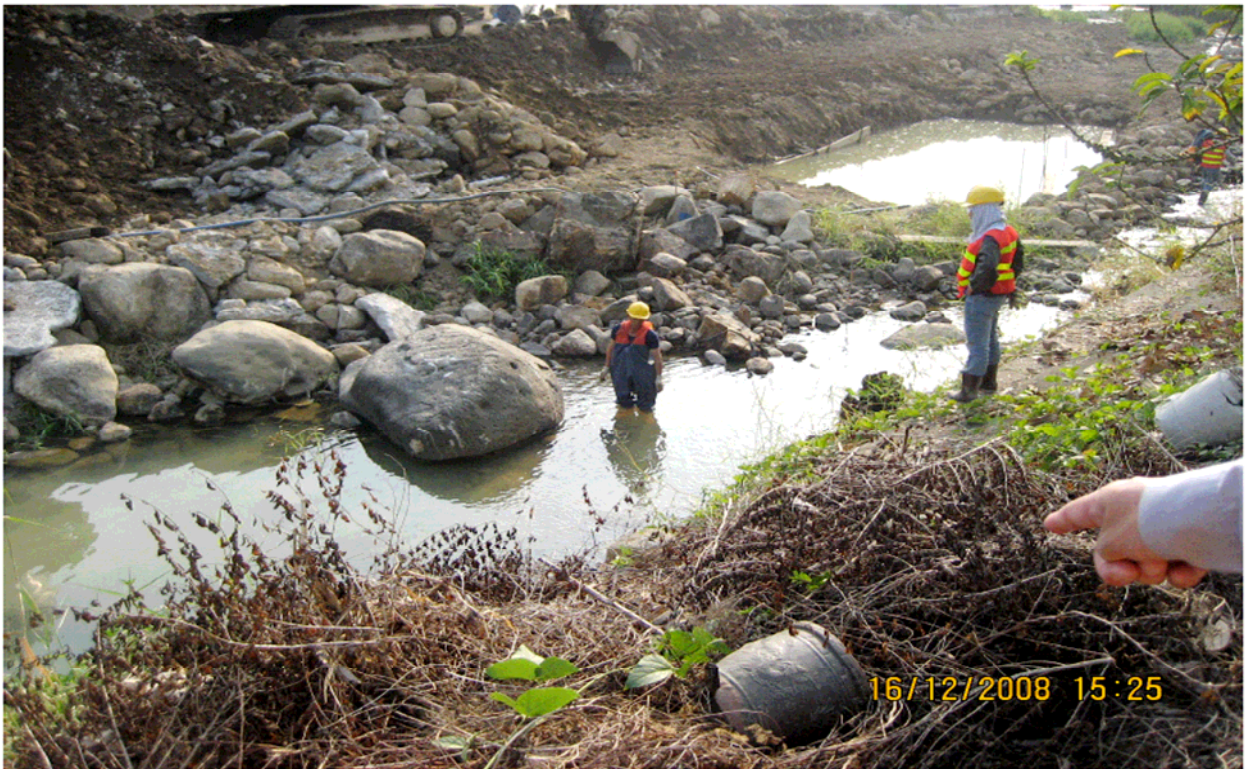
Fig.3 Disturbed riverbed from works carried out by site staffs
