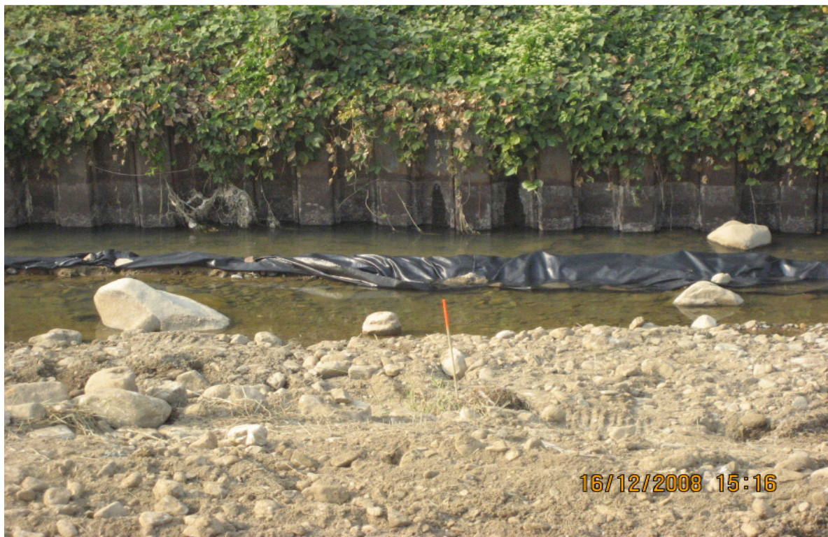
Fig.6 Insufficient height of barrier bunds at LTR
