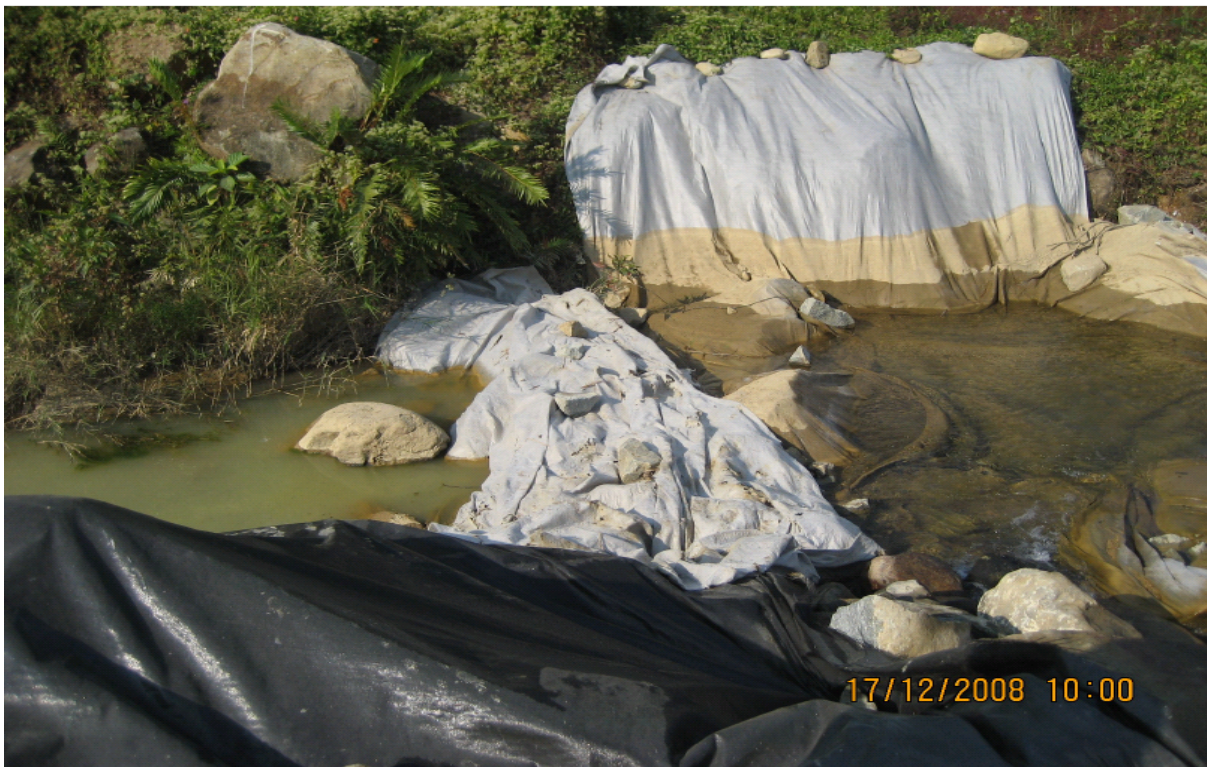
Fig.8 muddy water was being entered the river channel, located ch.100 of UTPR approximately
