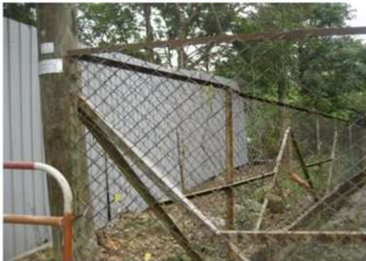
Fig.7.3 - Noise barriers have been relocated for protection to nearby sensitive receivers (photo taken on 1 st April)
