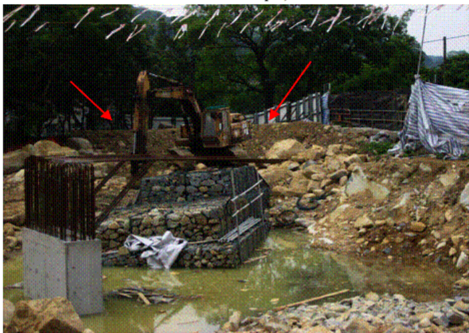
Fig.7.1 – Temporary noise barriers have been erected for noise protection (photo taken on 1 st April)
