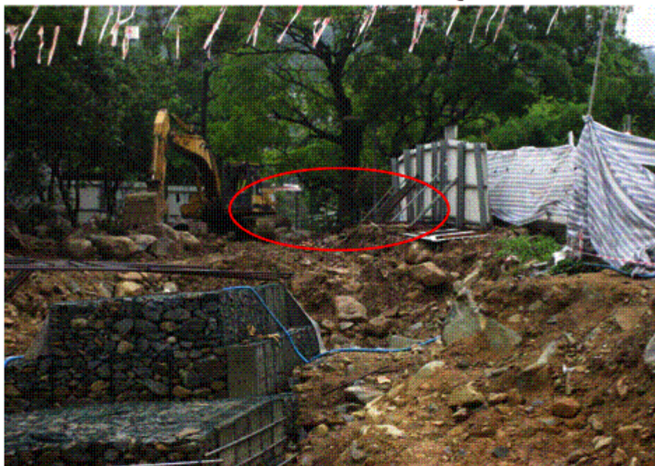
Fig.1 – Some of the sections without erection of noise barriers (photo taken on 25 th March)
