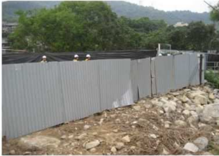
Fig.7.2 – Noise barriers have been relocated for protection to nearby sensitive receivers (Photo taken on 1 st April)
