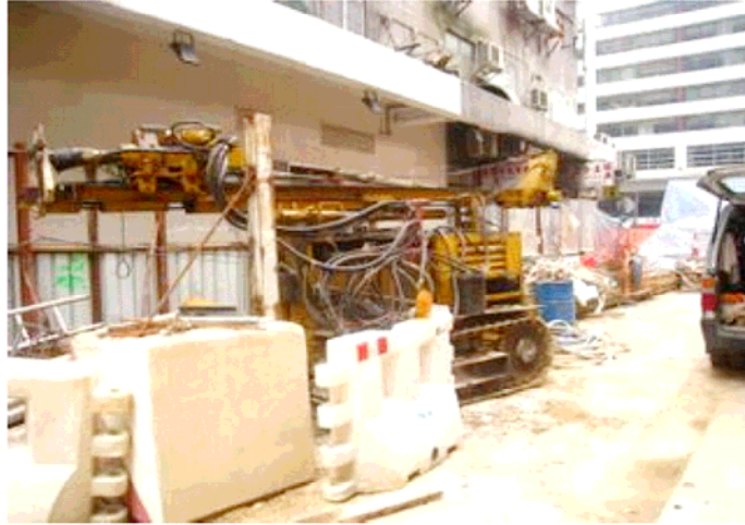
(Fig.3) The contractor relocated the operation rig during the follow up site inspection on 1 st April 2009.
