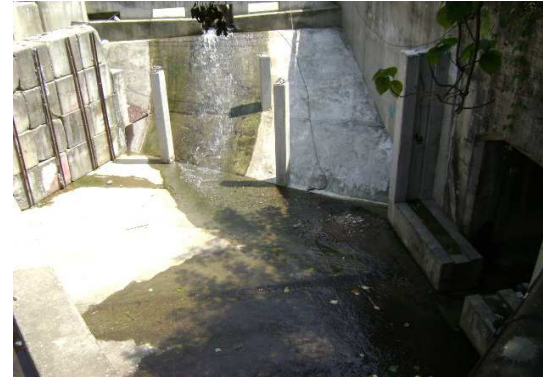
Photographic record for exceedance of Suspended Solids (SS) recorded at Sik Sik Yuen Ho Fung College (I-1) on 28-Sep-12
