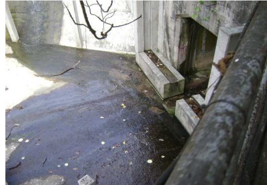
Photographic record for exceedance of Suspended Solids (SS) recorded at Sik Sik Yuen Ho Fung College (I-1) on 05-Nov-12
