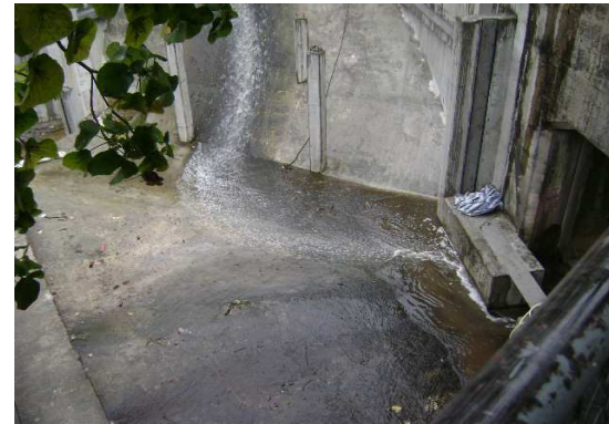
Photographic record for exceedance of Turbidity recorded at Sik Sik Yuen Ho Fung College (I-1) on 29-Dec-12
