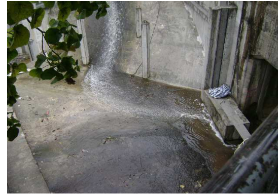
Photographic record for exceedance of Suspended Solids (SS) recorded at Sik Sik Yuen Ho Fung College (I-1) on 29-Dec-12
