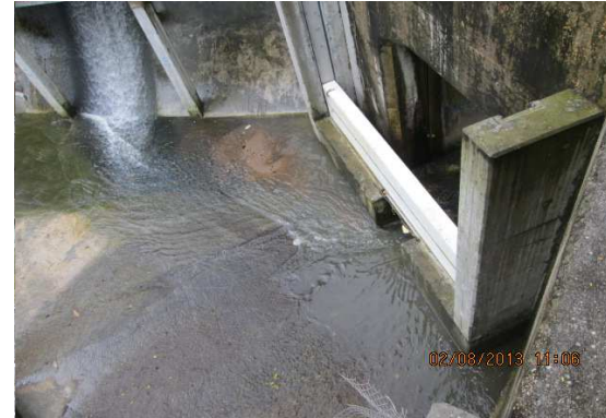
Photographic record for exceedance of Suspended Solids (SS) recorded at Sik Sik Yuen Ho Fung College (I-1) on 02-Aug-13
