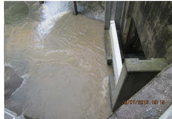
Photographic record for exceedance of Suspended Solids (SS) recorded at Sik Sik Yuen Ho Fung College (I-1) on 26-Jul-13
