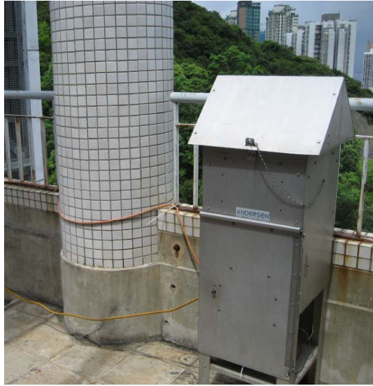
Air Quality Monitoring Station (AM1)
