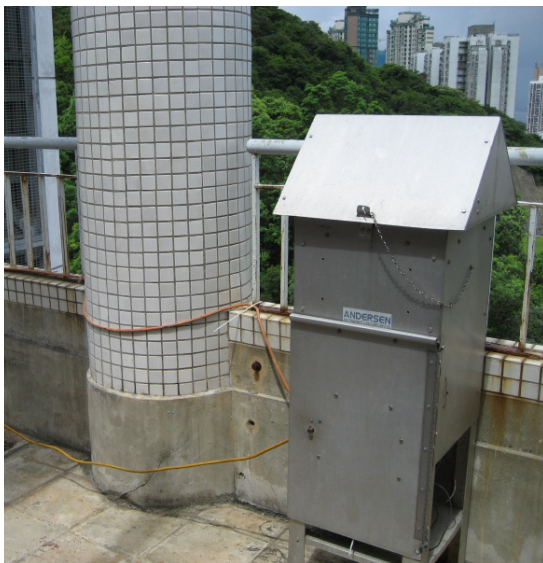
Air Quality Monitoring Station (AM1)
