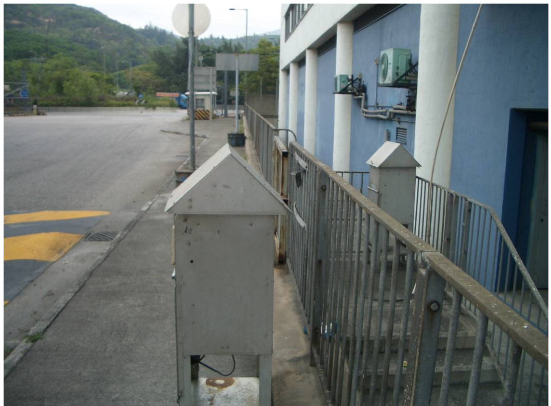
AM2 - River Trade Terminal Office
