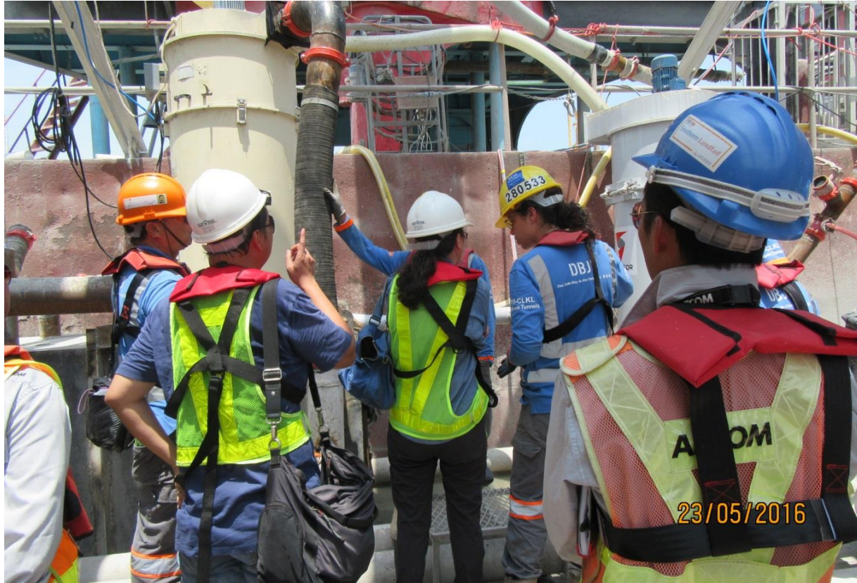
A joint site inspection was carried out by the ET, the Contractor, SOR and EPD on 23 May 2016. (Barge area - Southern Landfall)
