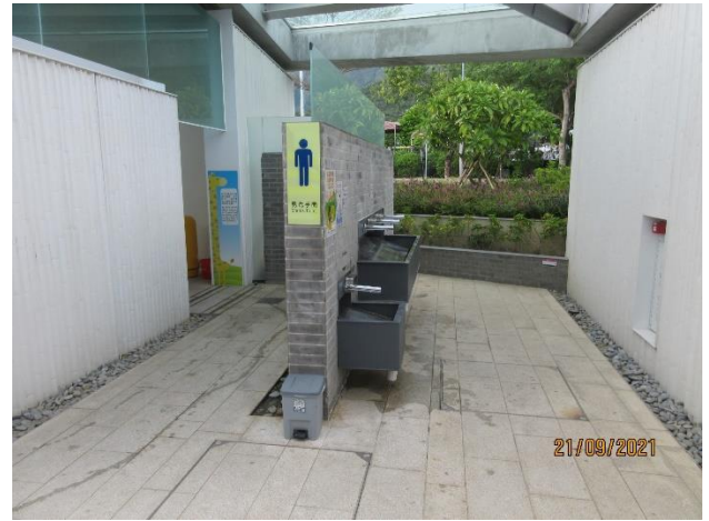
No plant in the planter outside the male (Planter P14) changing room
