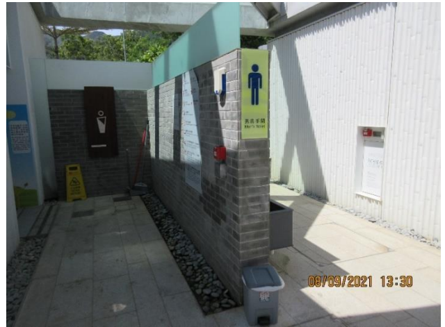
No plant in the planter outside the male (Planter P14) changing room
