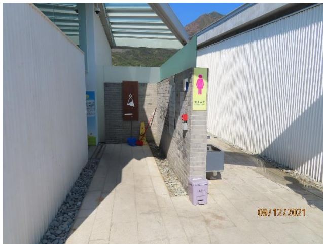
No plant in the planter outside the female (Planter P3b) changing room
