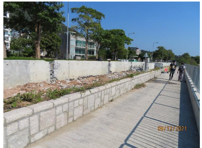
Plants at the Eastern box culvert were damaged by the concrete debris from the construction works
