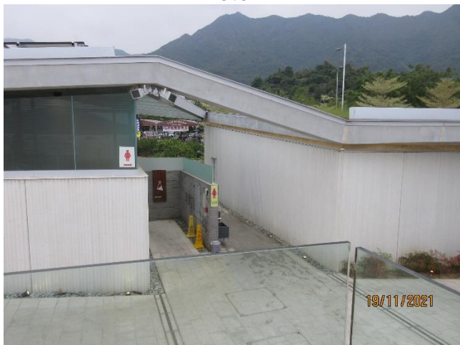
No plant in the planter outside the female (Planter P3b) changing room
