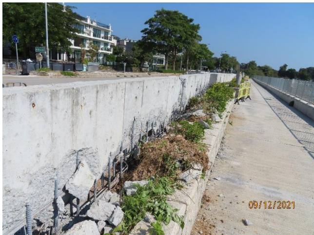
Plants at the Eastern box culvert were damaged by the concrete debris from the construction works
