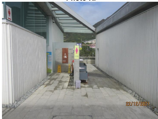
No plant in the planter outside the female (Planter P3b) changing room
