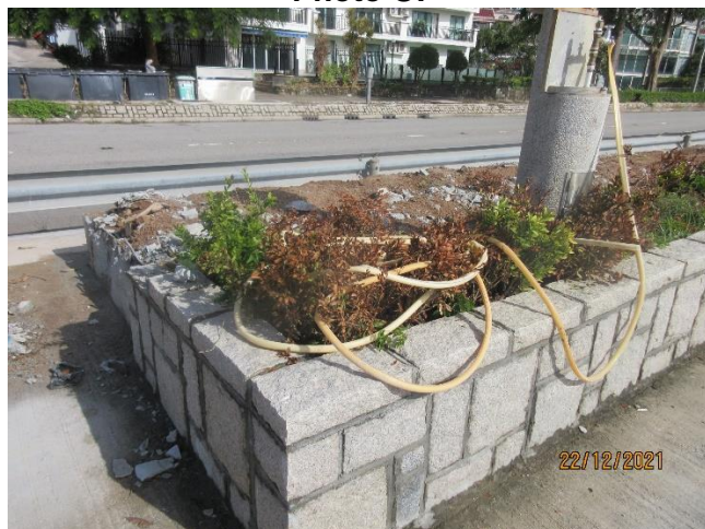
Plants at the Eastern box culvert were damaged by the concrete debris from the construction works
