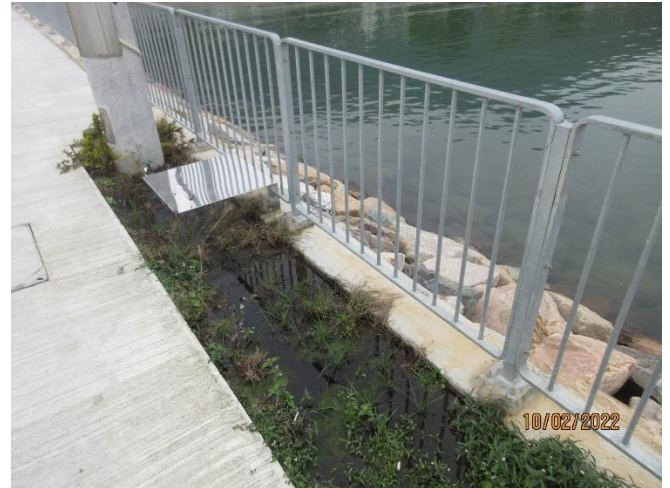
Poor soil drainage is found in one planter in Eastern Groyne
