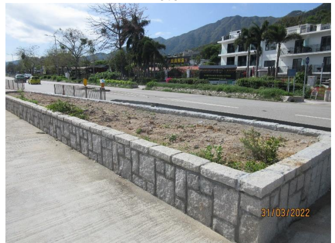
The planters at the Eastern box culvert were repaired and enlarged and the plants in the planters were removed
