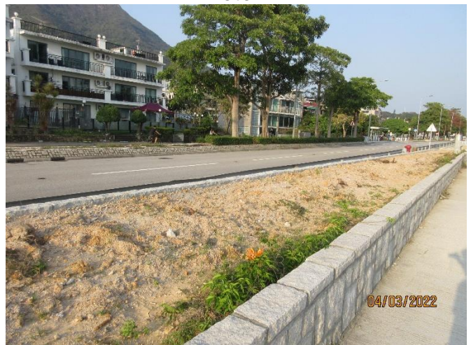
The planters at the Eastern box culvert were repaired and enlarged and the plants in the planters were removed
