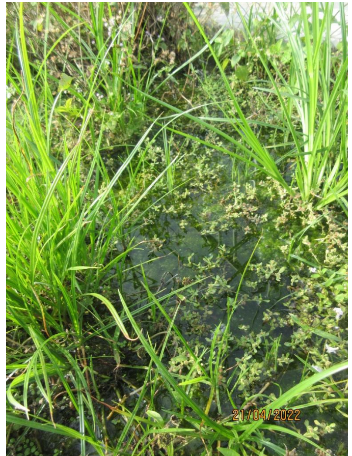
Poor soil drainage is found in one planter in Eastern Groyne
