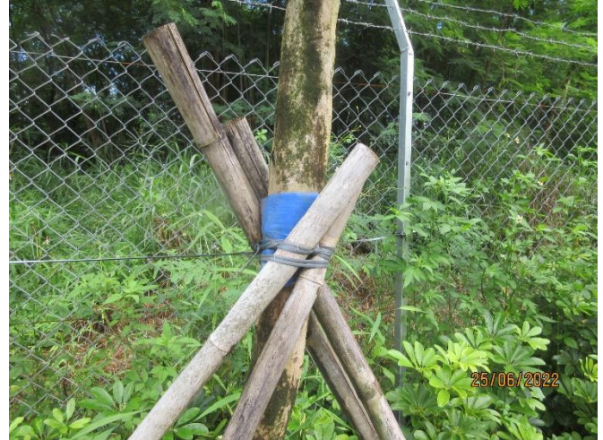
Some ties and stakes already girdled and affected the growth of the trees. Some unnecessary ties are attached between the trees.
