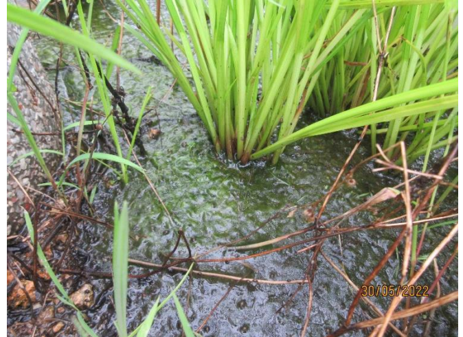
Poor soil drainage and serious water logging is found in one planter on the Eastern groyne.
