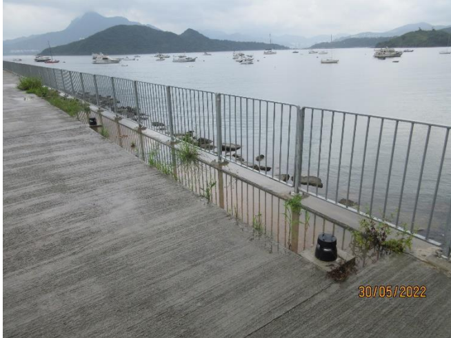
Some of the plants in the planters on the Western groyne were wilted and removed.
