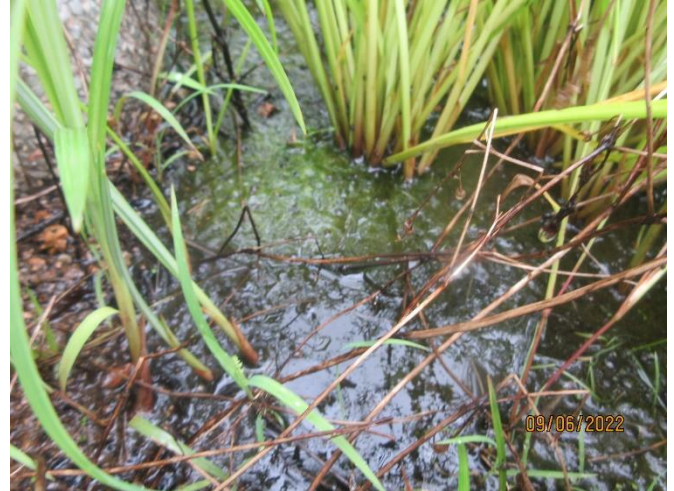
Poor soil drainage with water logging is found in one planter on the Eastern groyne.
