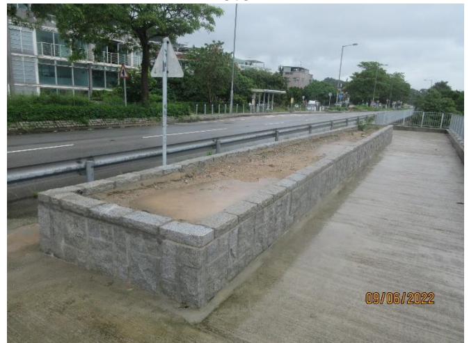
No plants in the Eastern box culvert planters.
