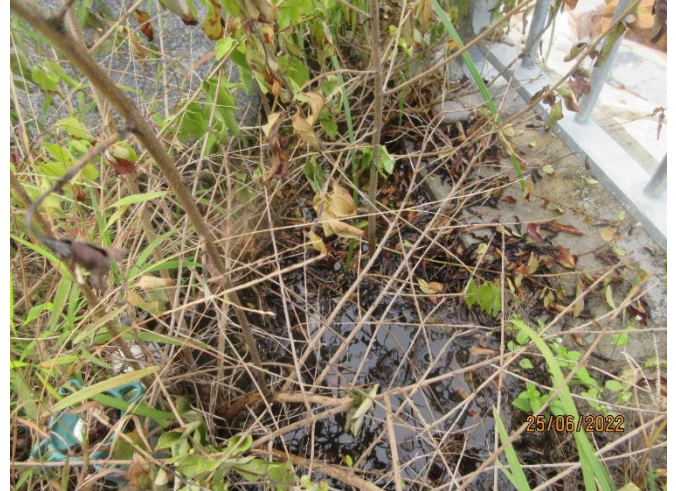
Poor soil drainage with water logging is found in one planter on the Eastern groyne.
