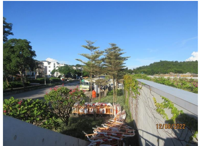
The Railing & debris damage the planters at the planter near Ting Kok Road
