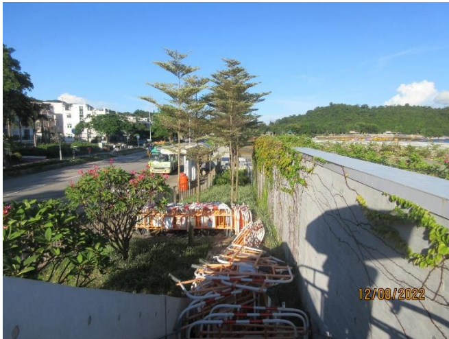
The Railing & debris damage the planters at the planter near Ting Kok Road
