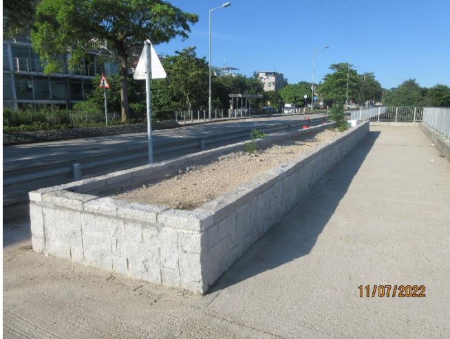
No plants in the Eastern box culvert planter.
