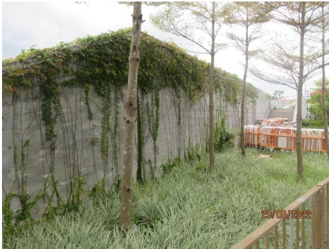
The Railing & debris damage the planters at the planter near Ting Kok Road
