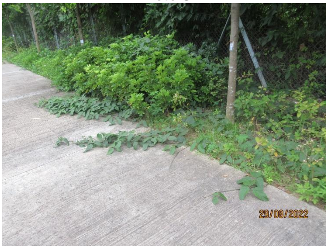
Some Pueraria sp. were found in planters and extending to footpath in the Western box culvert.
