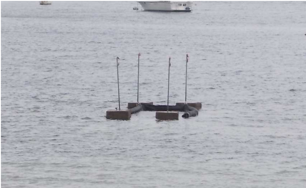
Photo 3. Demonstration of the fencing structure with concrete blocks and silt curtain in water
