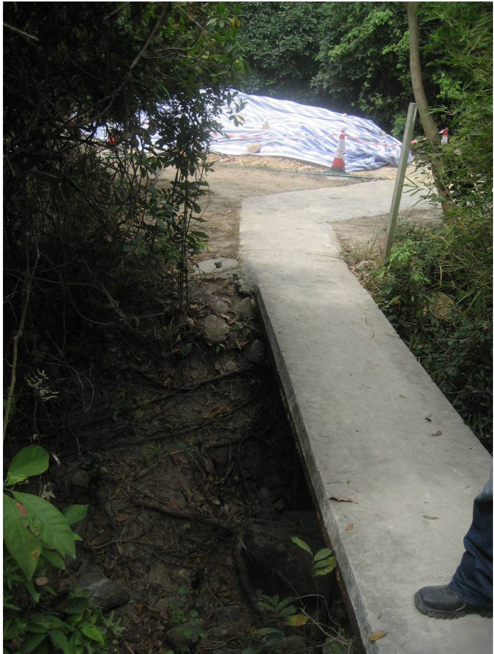
Photo 1 - Temporary stockpile was observed located next to the stream.
