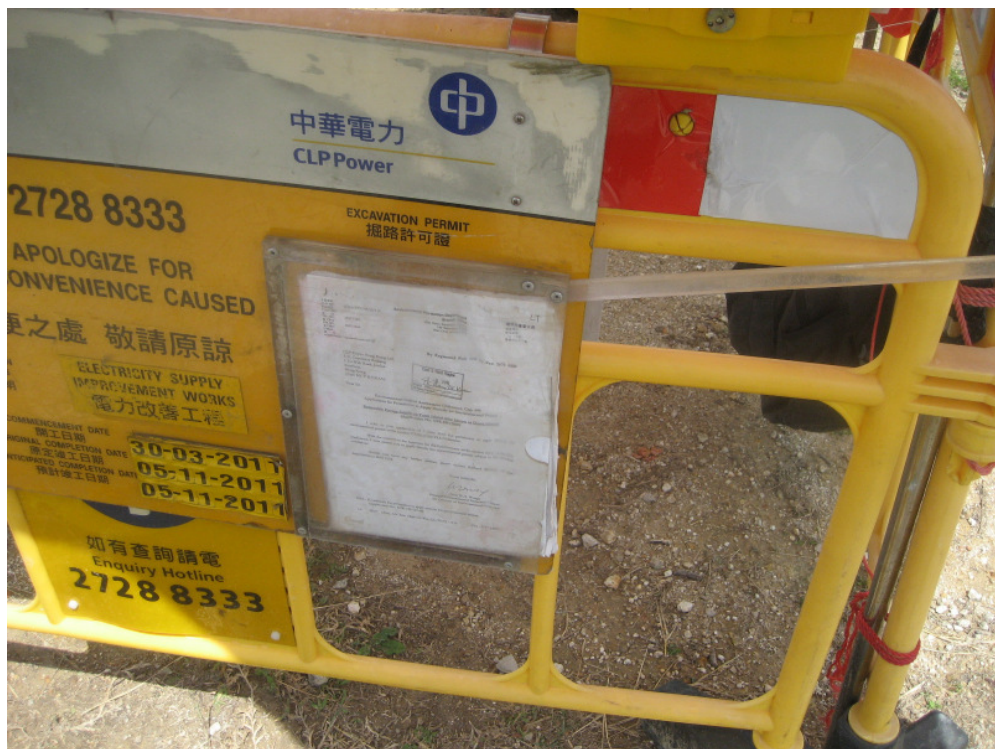
Photo 1 - The environmental permit and other documents were too thick and could not be taken out from the box folder.
