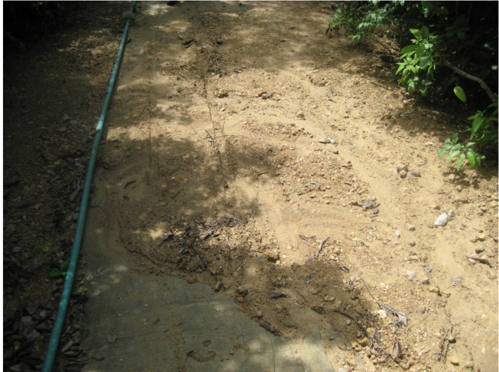
Photo 3 – Erosion was observed at the worksite for underground pipe and cabling works and eroded soil was accumulated at low-lying area.
