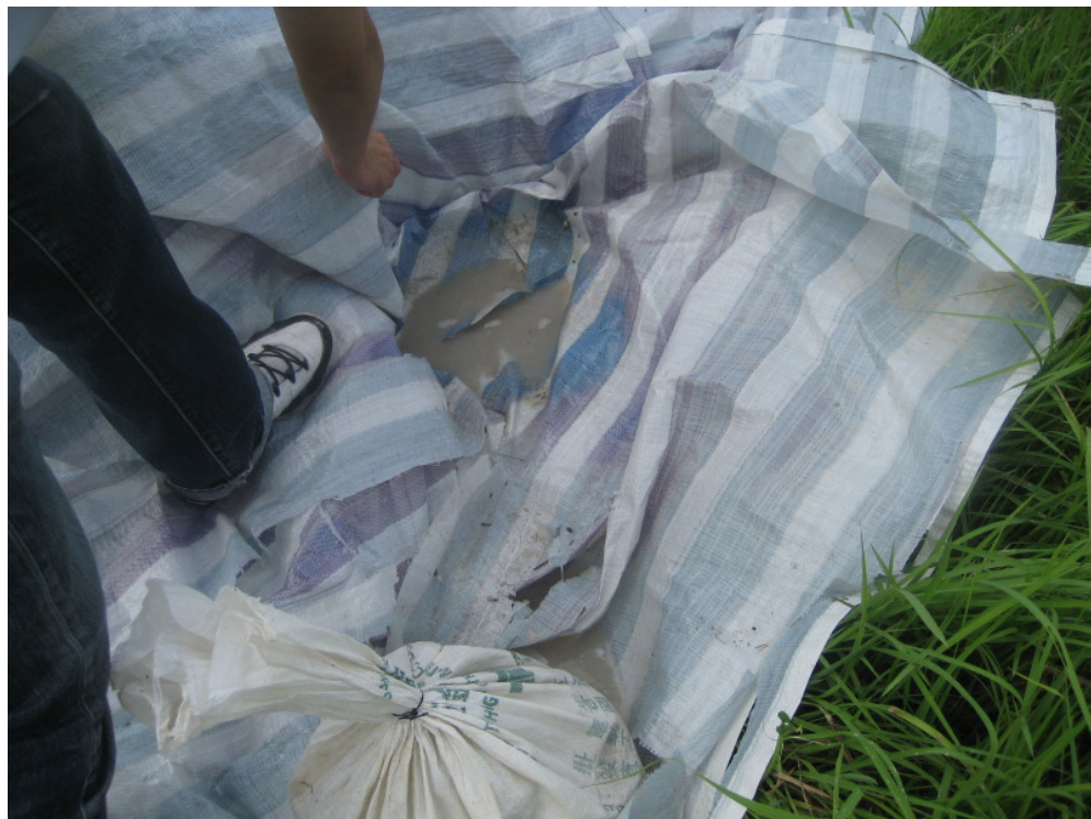
Photo 2 - Stagnant water was observed on the tarpaulin sheet covering the stockpile located at Site 1.
