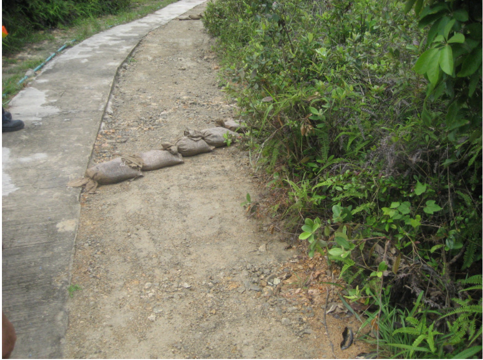
Photo 3 - Sand bags have been added at the worksite for underground pipe and cabling works to act as silt trap to prevent eroded soil from being washed away to low-lying areas.
