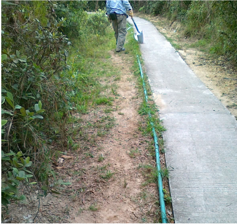
Photo 5 – The paint marking on soil and grassland at the temporary worksite for underground pipe and cabling works has been removed and the work sites has been reinstated.
