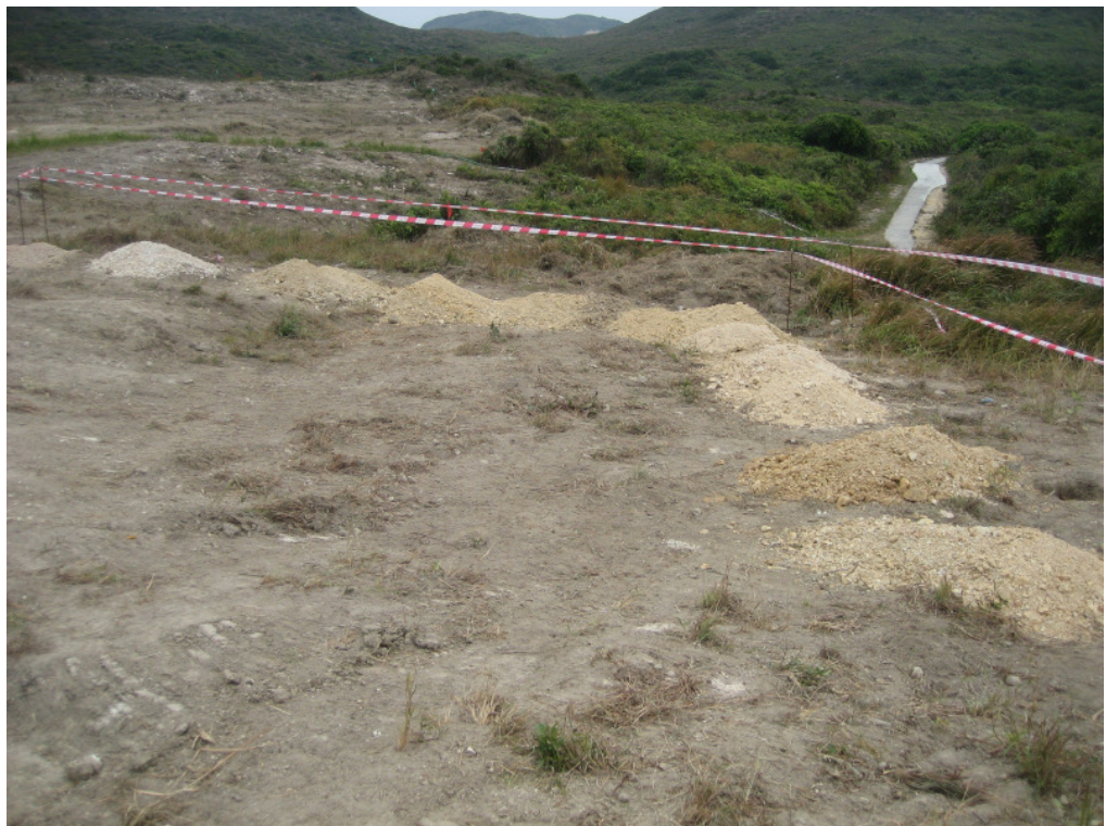
Photo 2 – The excavated material was observed not being covered at Site 1.
