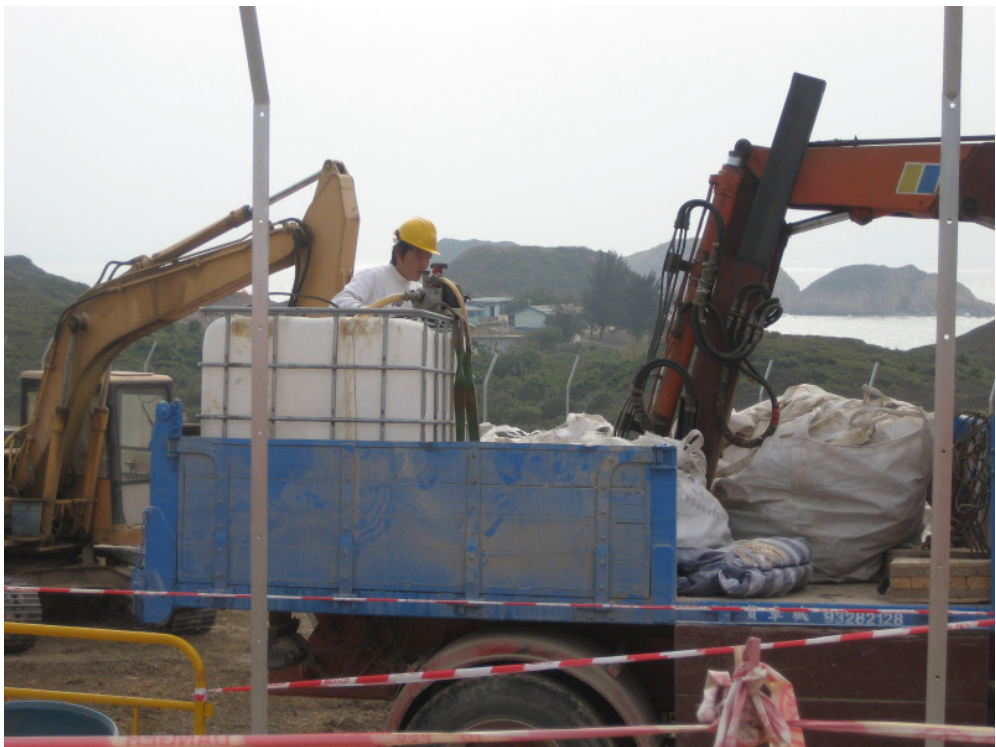
Photo 4 – Regularly wetting the exposed surface of the site has been done by the Contractor.
