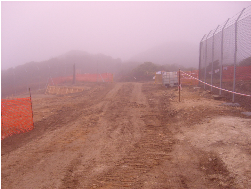
Photo 4 – Water tank has been provided at exit of Site 1 for washing the wheels of trucks leaving the construction site.
