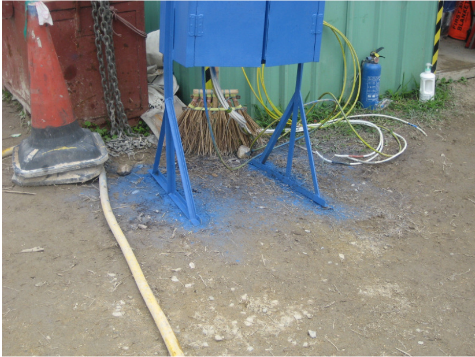
Photo 1 – Painting stain was observed on ground at Site 1.
