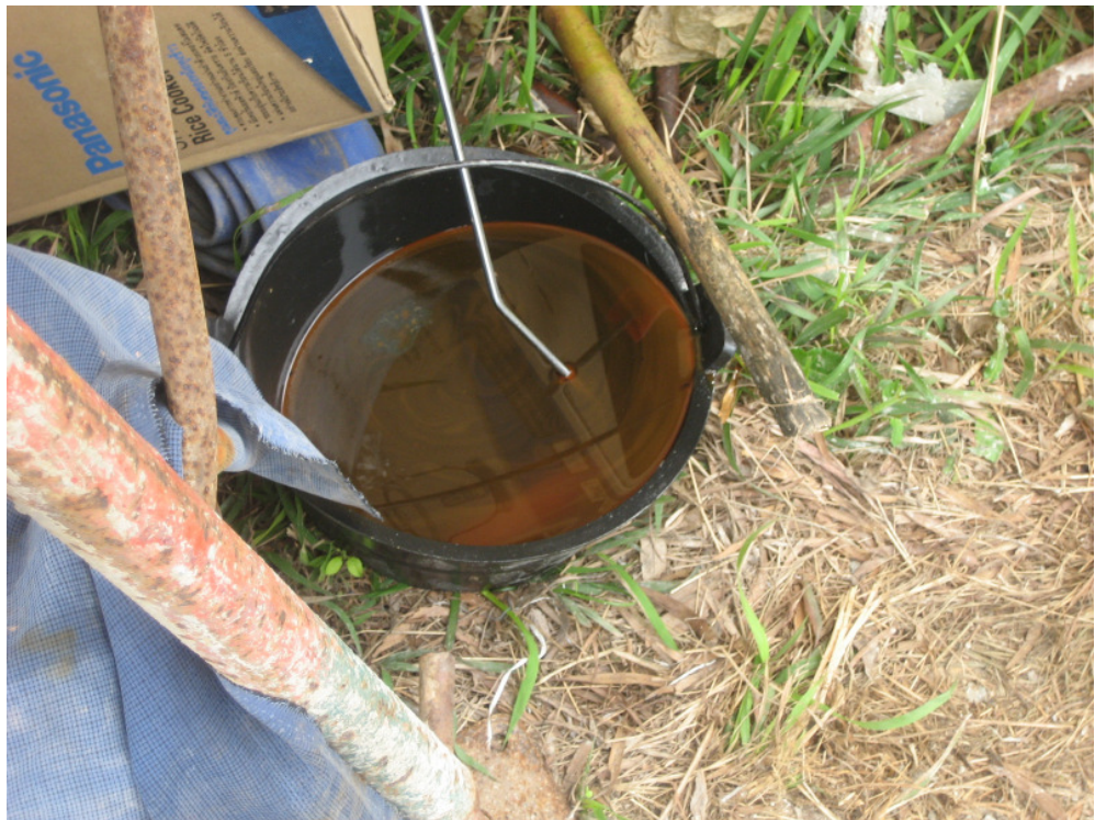
Photo 4 – Bucket with chemical was observed storing without cover and drip tray. Spillage was observed next to the bucket.
