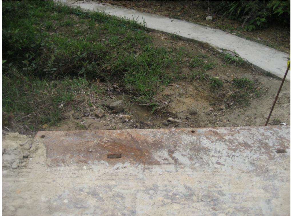
Photo 3 – The haul road crossing the stream was observed without earth bund.
