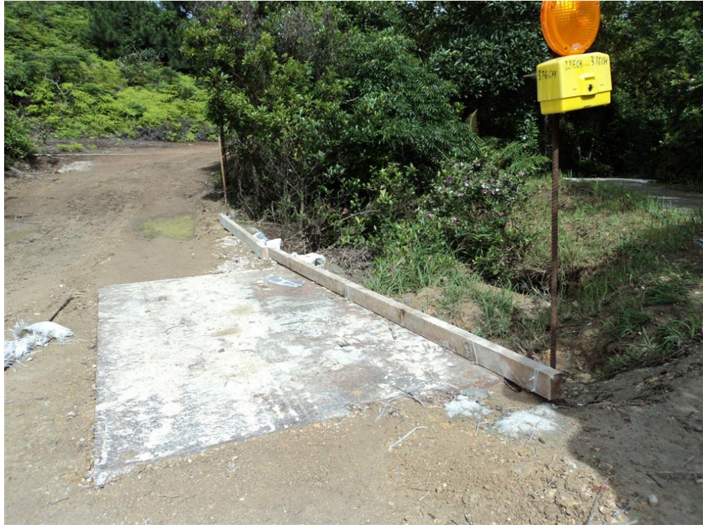
Photo 3 – A bund has been provided for the haul road crossing the stream.
