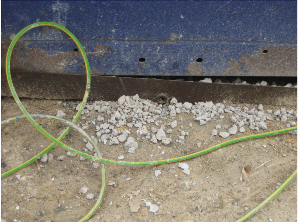
Photo 1 – Drip tray for the generator at Site 1 was observed with a hole being un-plugged.
