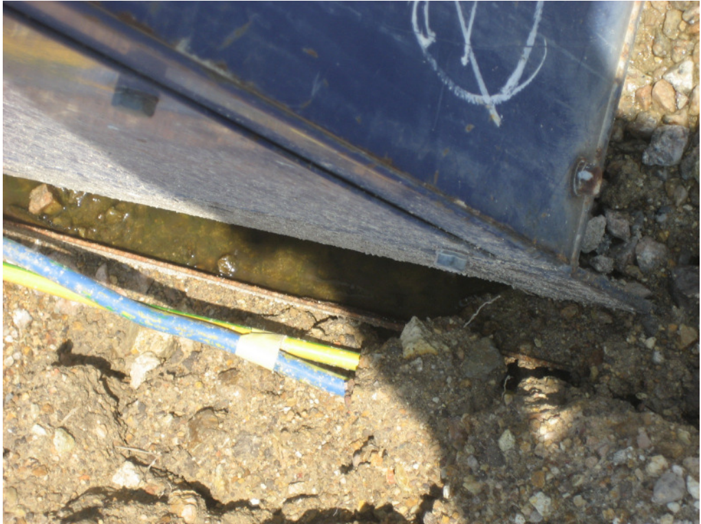
Photo 1 – Stagnant water in the drip tray under the generator at Site 1.
