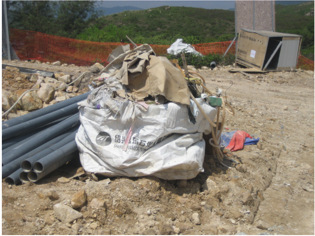
Photo 2 – General refuse was not properly stored at the designated area.
