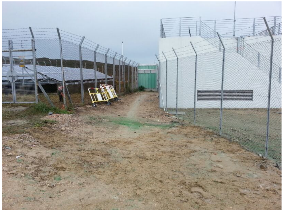
Photo 2 –Chemical stain had been removed following notification.
