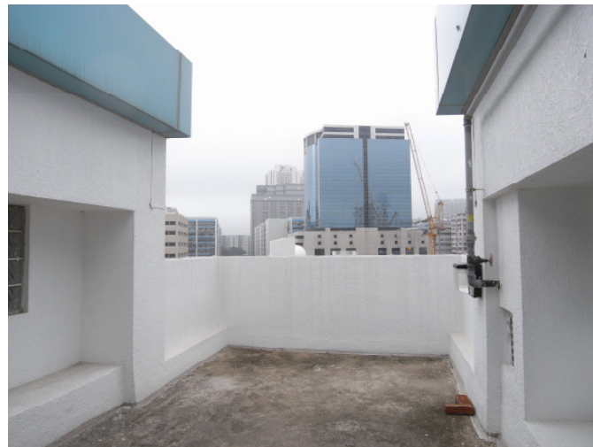
Monitoring location at KTSS
