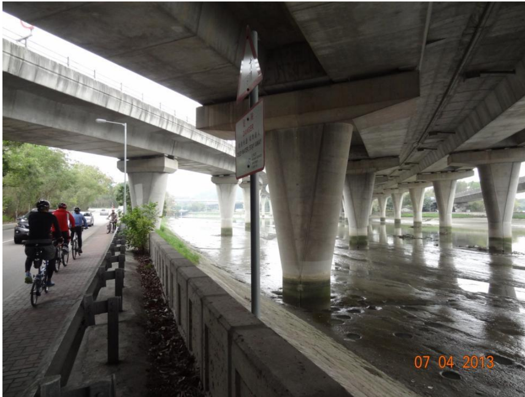
Location: (Section 1) Castle Peak Road (Tam Mi). Section underneath Tsing Long Highway.
