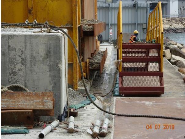
Earth bund was provided at the site boundary to prevent muddy surface run-off leakage into the water body.
