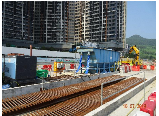
WetSept had been provided to treat any runoff water at Portion VI.
