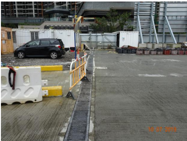
Cut-off drainage was provided at the site boundary to prevent muddy surface run-off leakage into the water body.
