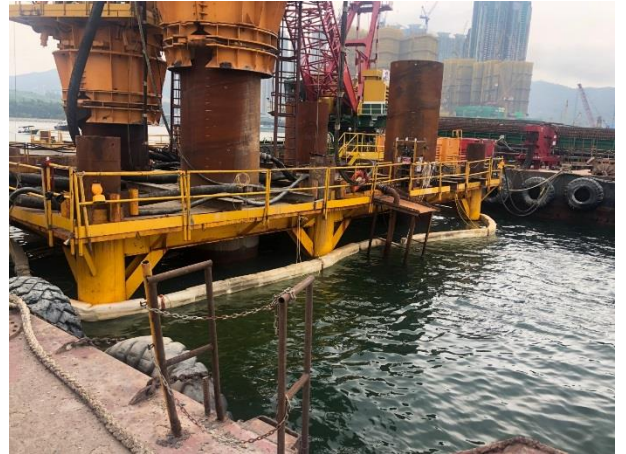
Silt curtain was installed to prevent the muddy water leakage into the water body.
