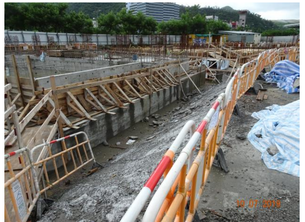
Concrete the exposed surface to reduce to create muddy water during rainstorm.
