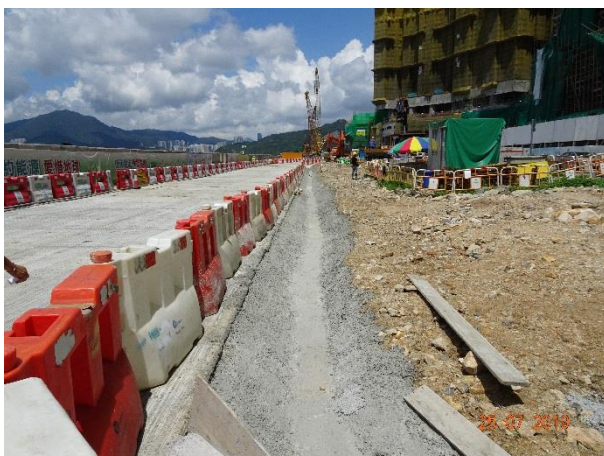
Part of the temporary drainage was installed to divert the site runoff to the de-silting facilities.
