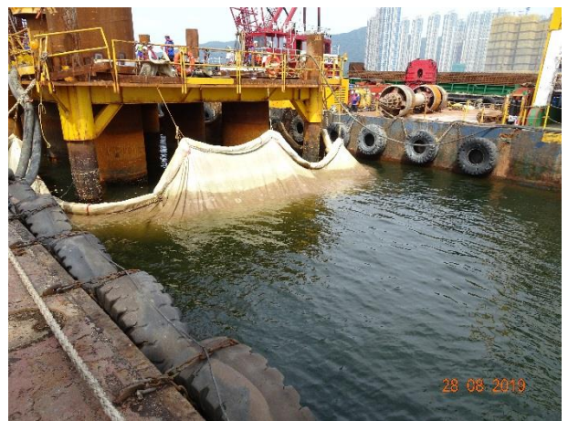
Silt-curtain had been provided to prevent muddy water overflow from the drilling platform.
