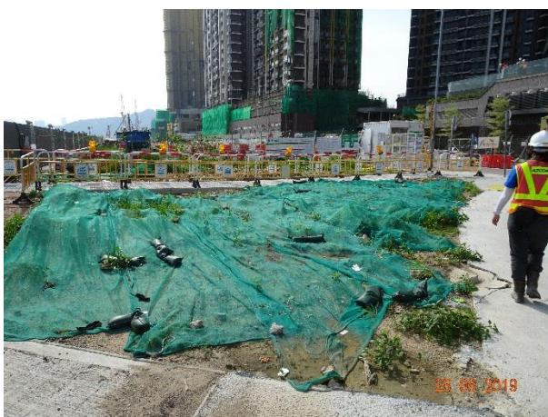
Using tarpaulin cover the exposed area to prevent generate turbidity runoff during rainstorm.
