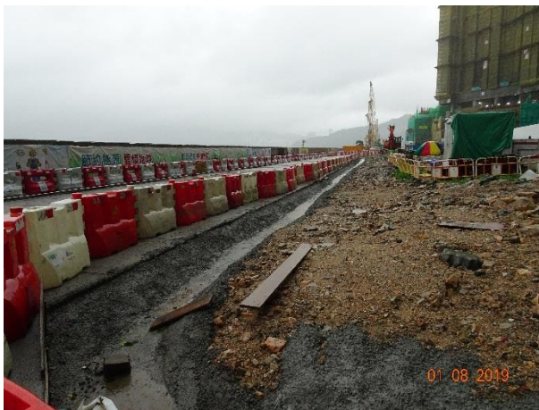
Part of the temporary drainage was installed to divert the site runoff to the de-silting facilities.
