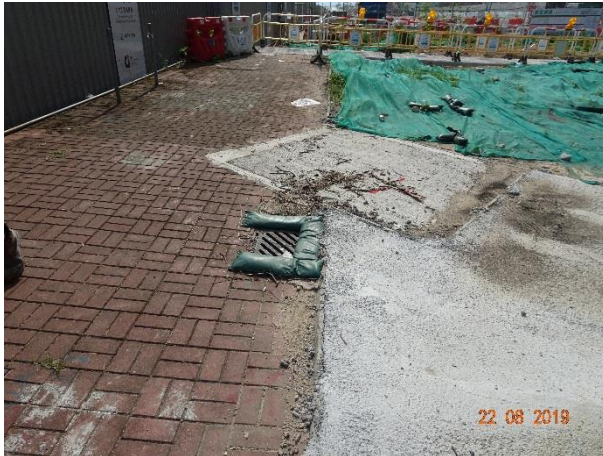
Sand bags had been provide to prevent site runoff overflow to the existing manhole.
