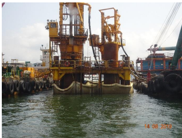
Silt-curtain had been provided to prevent muddy water overflow from the drilling platform.
