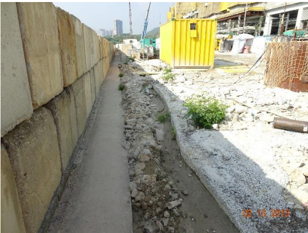
Trench had been installed beside the sea front to prevent muddy surface run-off overflow during rainstorm.
