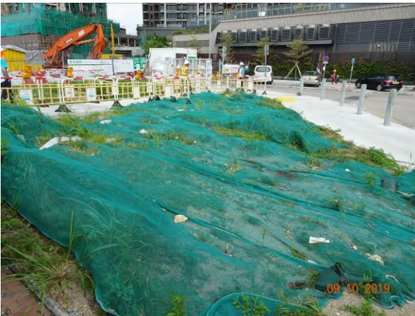
Exposed area had been covered to prevent muddy surface run-off during rainstorm.
