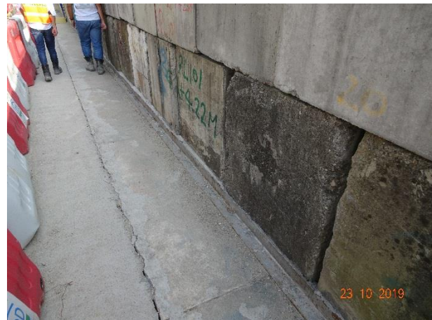
Gap between the concrete block and the sea front was sealed up.
