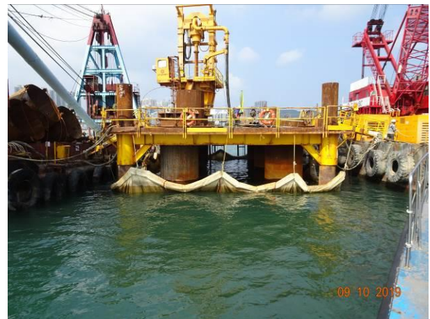
Silt-curtain had been provided to prevent muddy water overflow from the piling platform.
