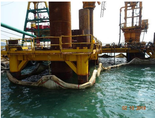
Silt-curtain had been provided to prevent muddy water overflow from the piling platform.
