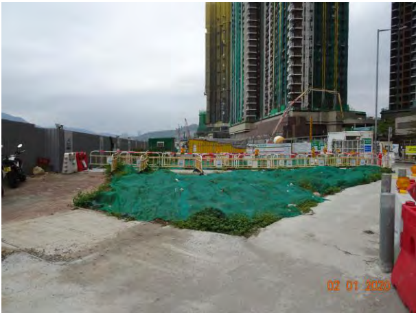
Exposed area had been covered to prevent muddy surface run-off generation during rainstorm.
