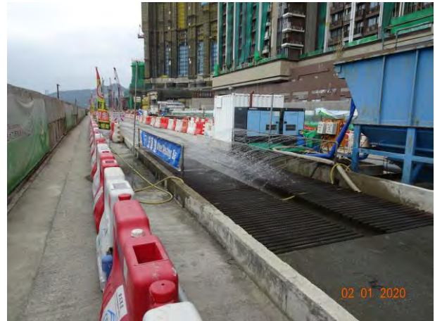
Treatment facilities was installed at site to treat the site generated water prior discharge.
