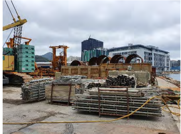
Temporary trench had been installed at the sea front to prevent muddy run-off overflow into the water body during
