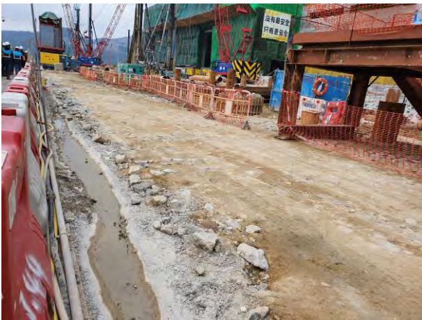
Trench had been installed beside the sea front to prevent muddy surface run-off overflow during rainstorm.
