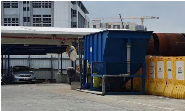
Treatment facilities was installed at site to treat the site generated water prior discharge.
