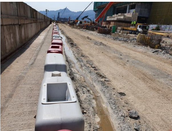
Trench had been installed beside the sea front to prevent muddy surface run-off overflow during rainstorm.
