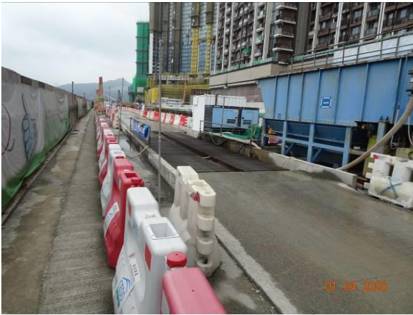
Treatment facilities was installed at site to treat the site generated water prior discharge.
