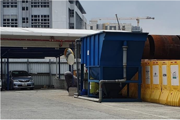
Treatment facilities was installed at site to treat the site generated water prior discharge.
