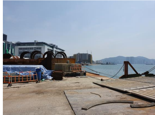
Temporary trench had been installed at the sea fount to prevent muddy run-off overflow into the water body during
