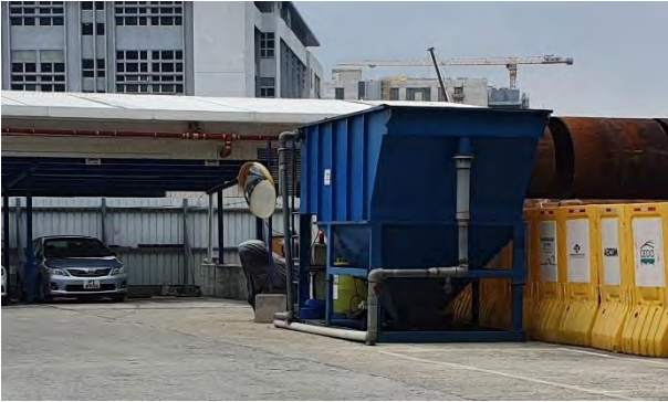
Treatment facilities was installed at site to treat the site generated water prior discharge.
