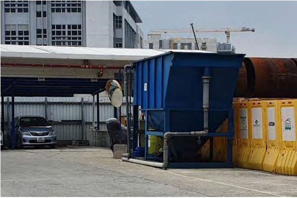
Treatment facilities was installed at site to treat the site generated water prior discharge.
