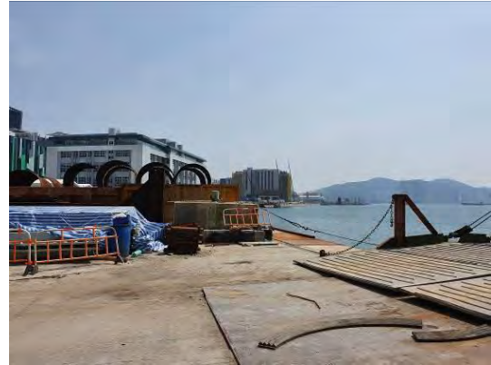
Temporary trench had been installed at the sea front to prevent muddy run-off overflow into the water body during
