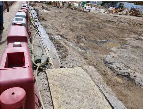
Trench had been installed beside the sea front to prevent muddy surface run-off overflow during rainstorm.
