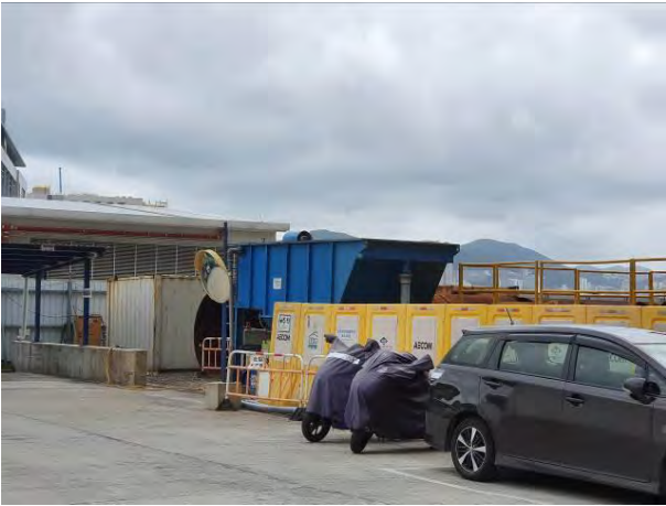
Treatment facilities was installed at site to treat the site generated water prior discharge.
