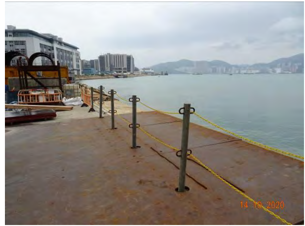
Temporary trench had been installed at the sea front to prevent muddy run-off overflow into the water body during rainstorm.
