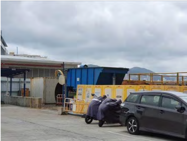
Treatment facilities was installed at site to treat the site generated water prior discharge.
