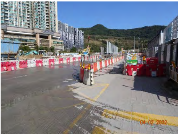
Treatment facilities was installed at site to treat the site generated water prior discharge.
