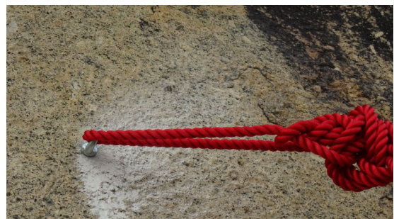
Installation of safe access facilities around the daylighting location on Sheung Sha Chau Island
