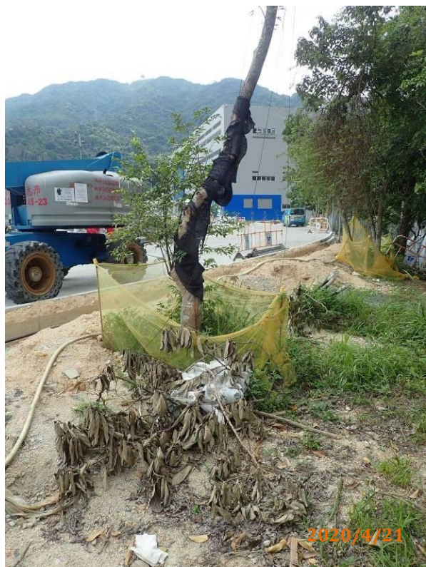
Photo 12. No equipment, waste, or construction materials shall leaning on plant protection zone. Collapsed fence shall be promptly rectified.
