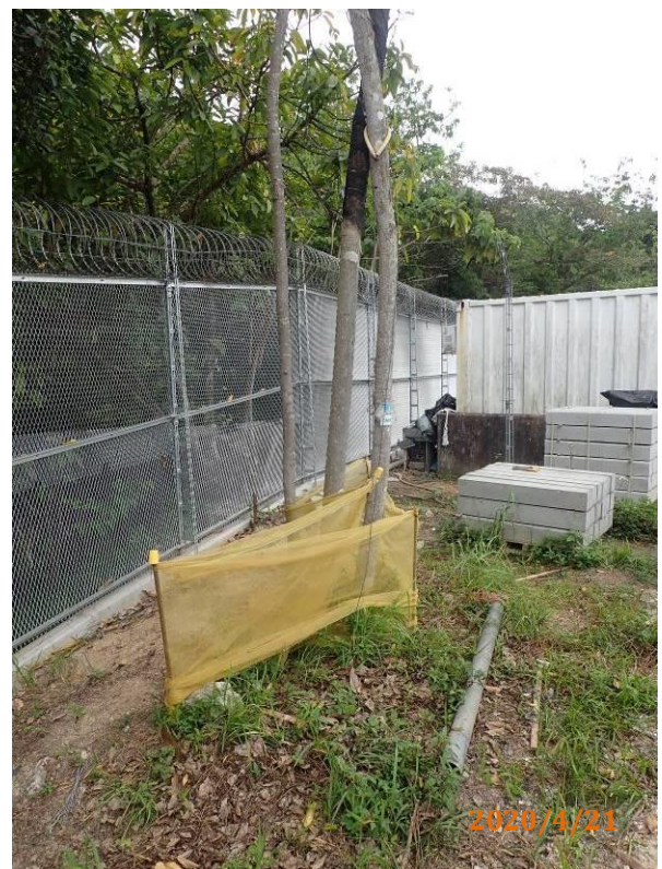
Photo 13. Collapsed fence shall be promptly rectified.
