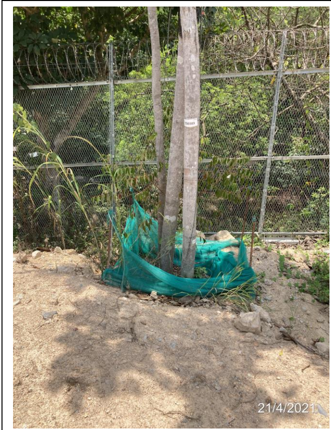
Photo 8. Collapsed fencing of TA572 to be rectified
