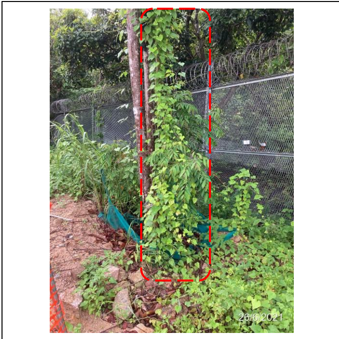
Photo 8. Collapsed fencing of TA572 to be rectified. The climbers on trunk shall be cleared.
