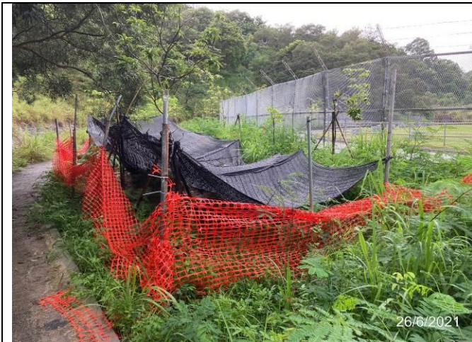
Photo 1. Collapsed shelter for Cibotium barometz to be rectified
