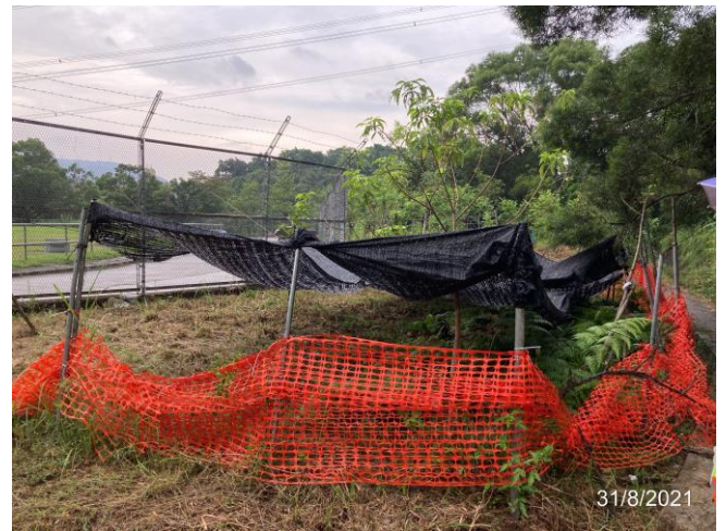
Photo 2. Collapsed fencing to be rectified
