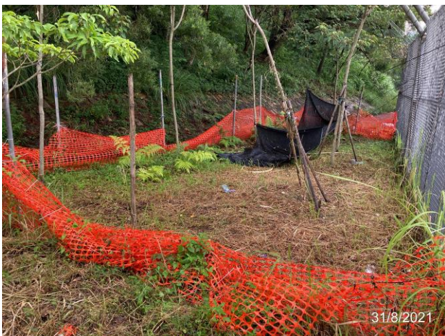
Photo 5. Collapsed shelter and fencing to be rectified
